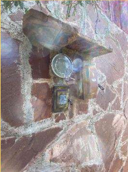
Very little electrical system components remain.
