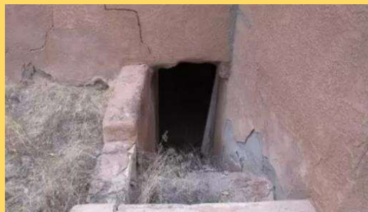
A steep set of exterior stairs lead down to the basement entrance
