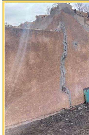
Evidence of settling causing bathroom addition to separate from main structure
