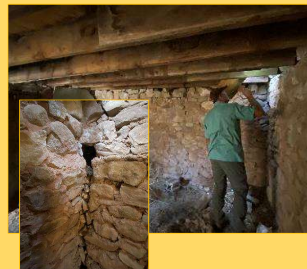
Photos of basement walls which create foundation for some of the walls above. These basement walls appear to be fairly intact and stable.
